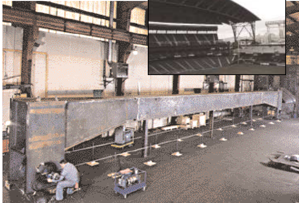
CPMT used the BB 5000 boring bar to perfectly align pivot holes 80 feet apart in four 85-foot sill beam segments, used in Safeco Field’s unique retracting roof (inset).
